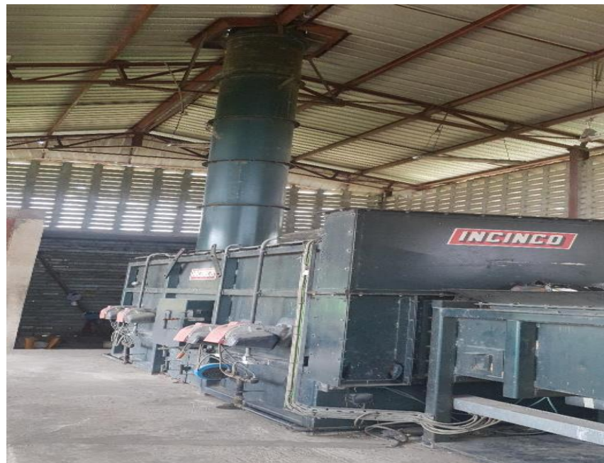
Figure 5. Waste incinerator at Petroleum Training Institute (PTI), Effurun, Nigeria.
